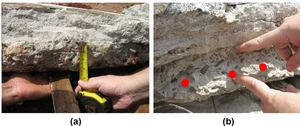
Fig. 5. (a) Excessive layers of mortar, filler and coating and (b) detail of the downgrade of the negative reinforcement and lack of uniformity for the spacing between bars.
