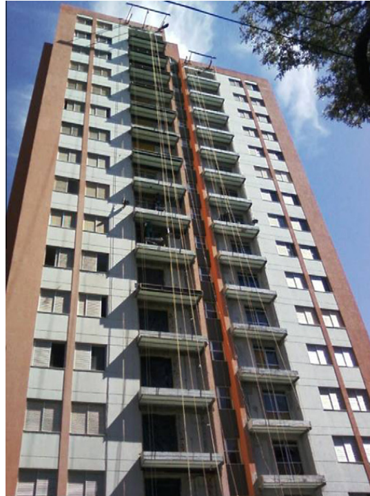
Fig. 12. Frontage of the damaged building after the reconstruction of the failed/demolished balconies.
