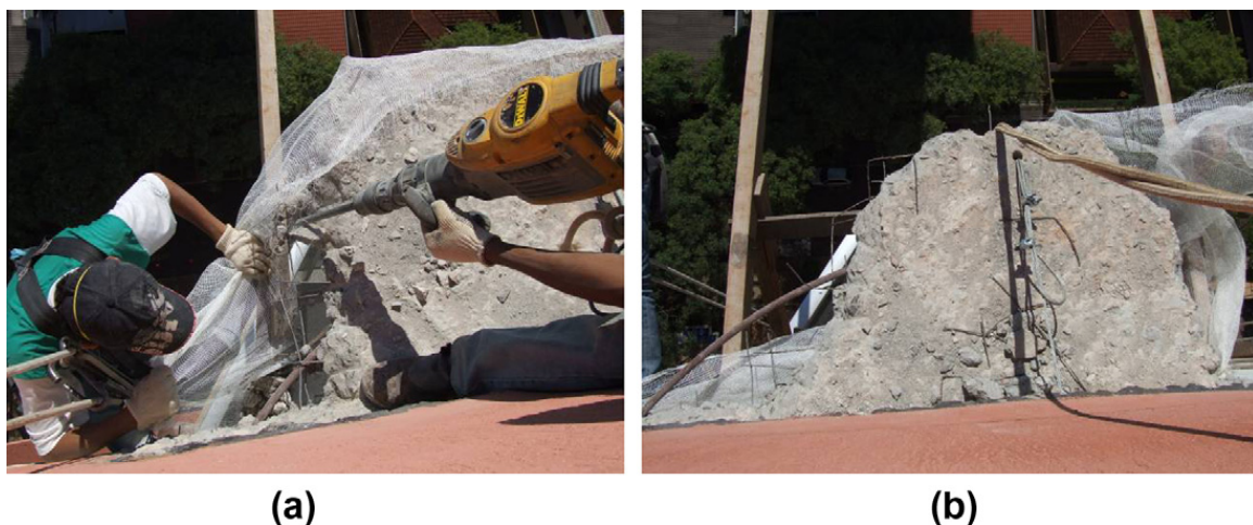
Fig. 7. (a) Free-stand slab being demolished using mechanical drill and (b) steel cables providing additional safety for the slab under demolition.
