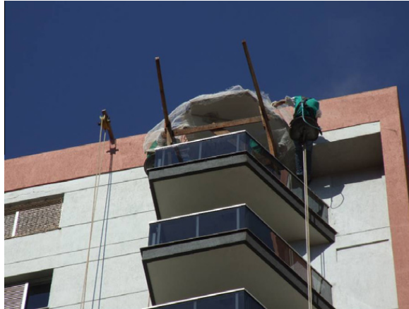
Fig. 6. Metal guides installed in the coverage of the building in order to suspend workers using safety belts connected to steel cables.
