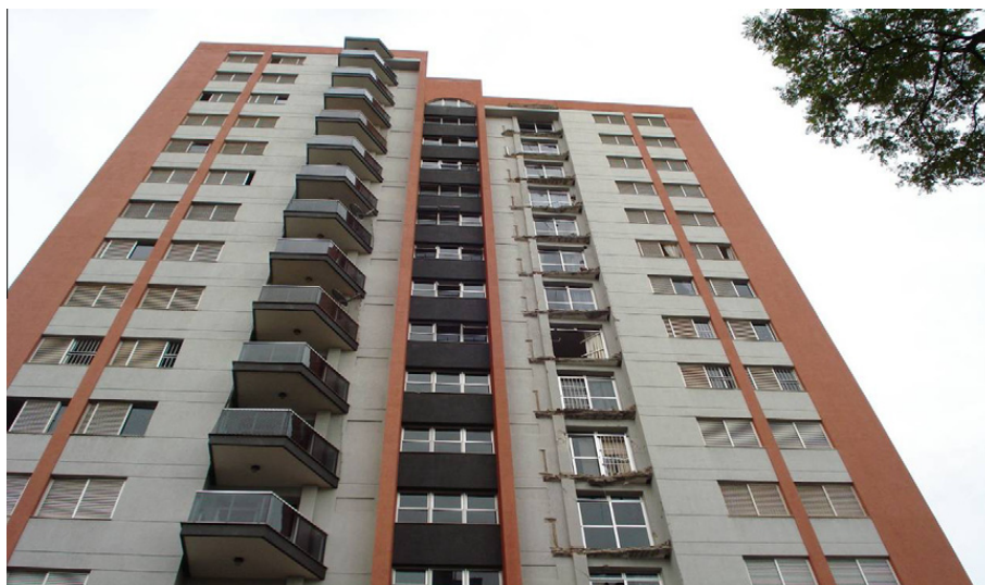
Fig. 1. Progressive failure of balconies of a housing building in Maringá (Brazil).
