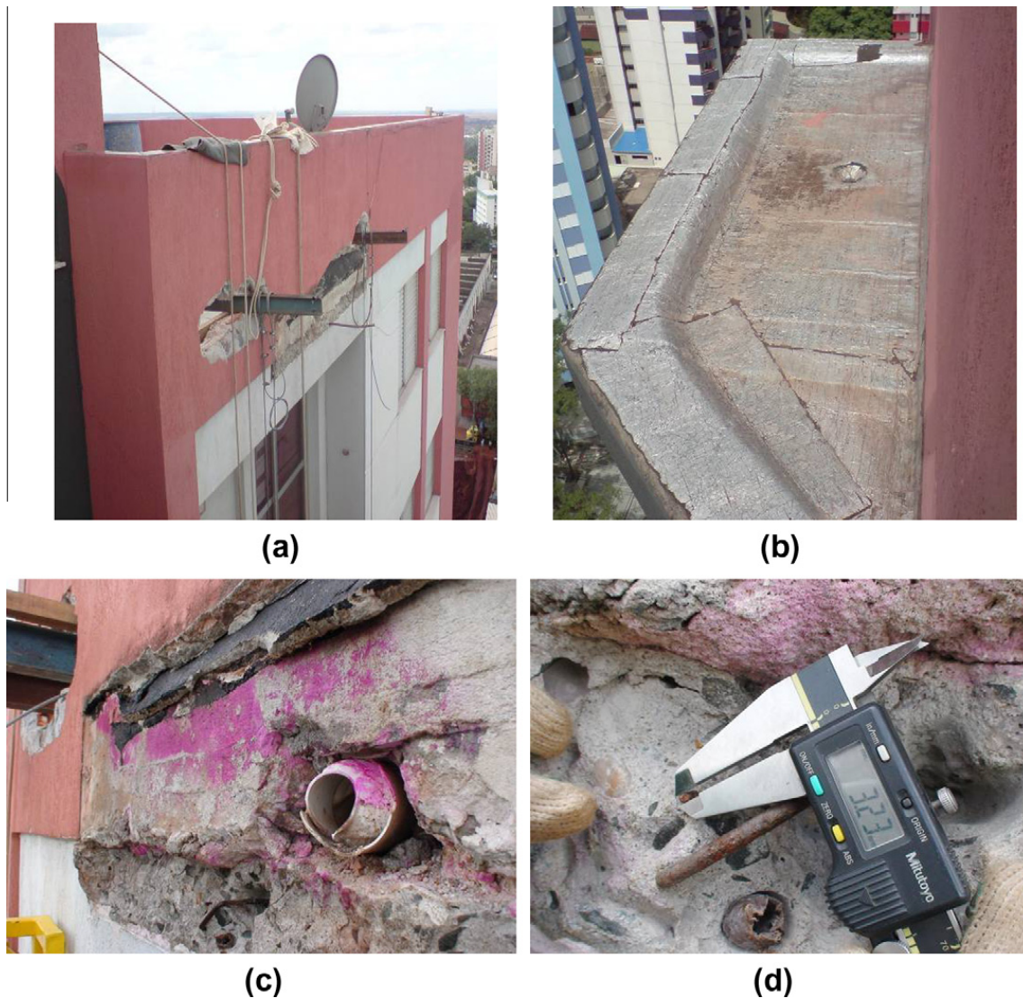
Fig. 4. (a) Details of the region of detachment of the canopy, (b) non-forecasted loadings acting on the reminiscent canopy, (c) simple test using phenolphthalein for showing a propitious region for corrosion, and (d) decreasing of the main negative bar in the failed canopy indicating corrosion.
