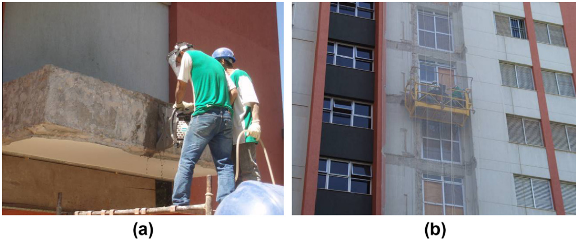
Fig. 8. (a) Reinforced concrete pot plant extracted using a diamond saw and (b) installation of a suspended working platform after removing all the reminiscent balconies.
